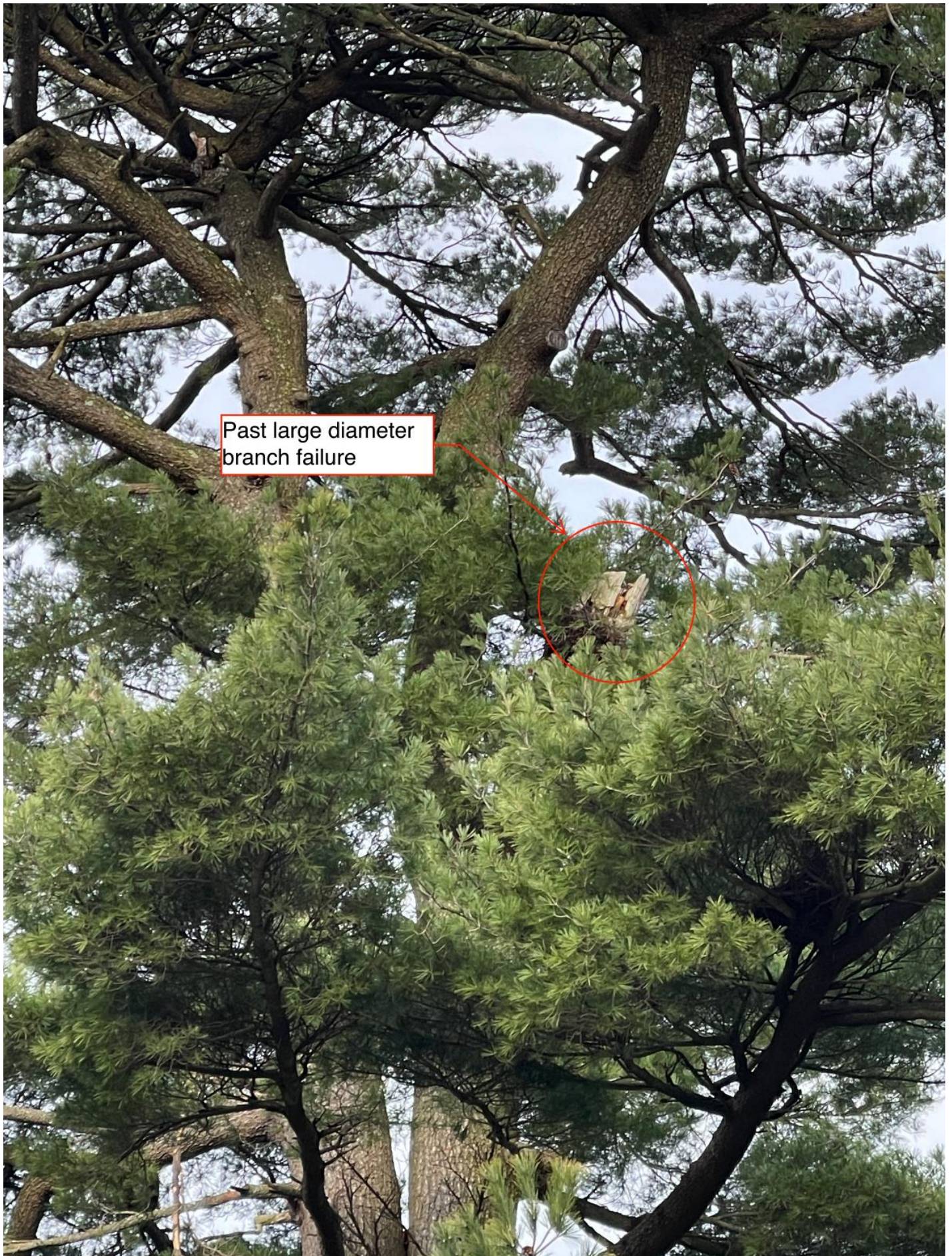
Potograph #10: Tree #2 Closeup of branch failure.
