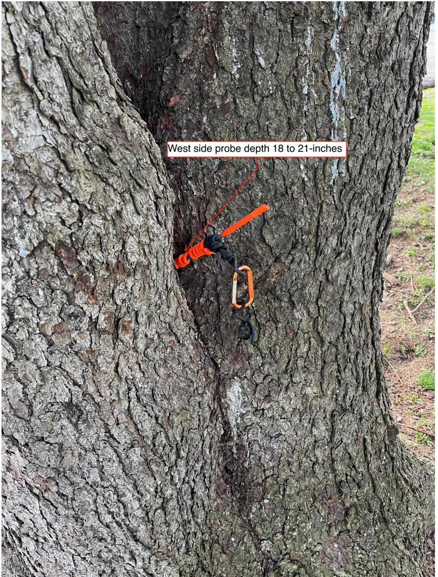
Photograph 5: Tree #1 Probe inserted into seam 18 to 21-inches on west side of tree.
